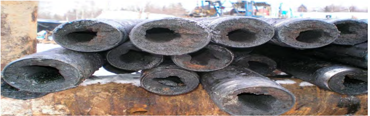
Fig.1.11: Oil and gas pipeline under sweet corrosion[62].
