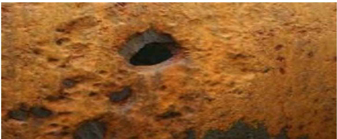
Fig.1.7: Pitting Corrosion of oil and gas pipeline [54].
