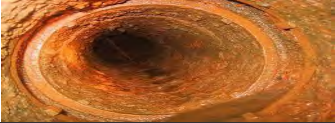
Fig.1.3: Internal Corrosion of oil and gas pipeline [46].
